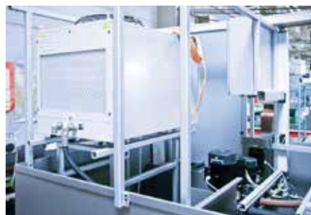
External cooling unit For temperature stability of machine and dielectric.
